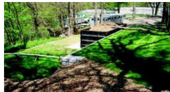
After receiving assistance and funding from the Council, this farm’s revised waste system now includes a retaining wall, convenient and safe dumpster access, and concrete pad that minimizes water quality issues, improves hauling access and ultimately saves the farm money..
